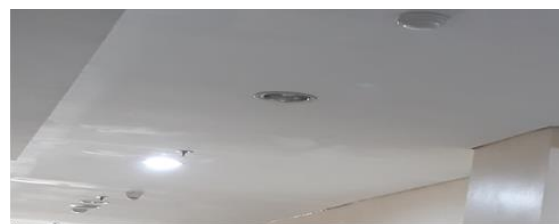
Gambar 5 Sprinkler RS Awal Bros
