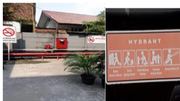
Gambar 6 Hydrant RS Awal Bros
